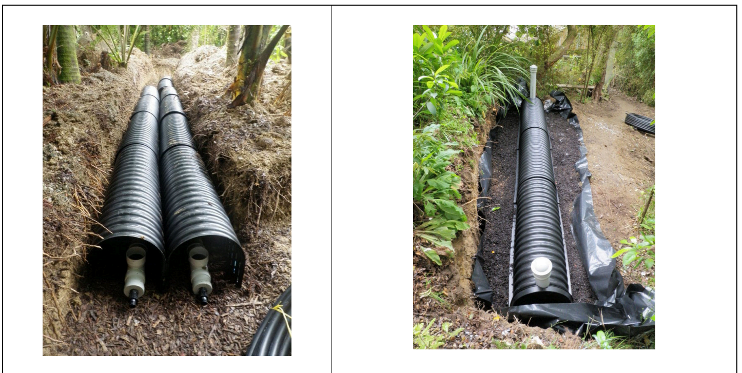
Figure 5. Examples of humus trenches under construction (from Mike Copeland, Kiwi Pioneer, Westport)
